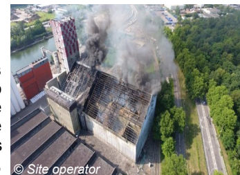
© Site operator Silo explosion linked to inappropriate management of concurrent activities (ARIA 51652)
