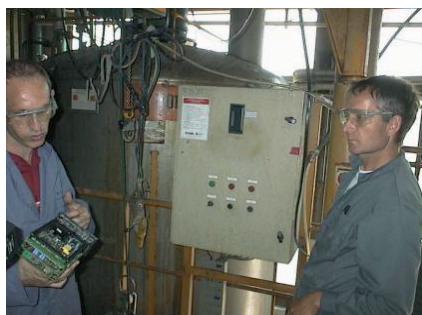
Failure of an automation controller card responsible for an accident
