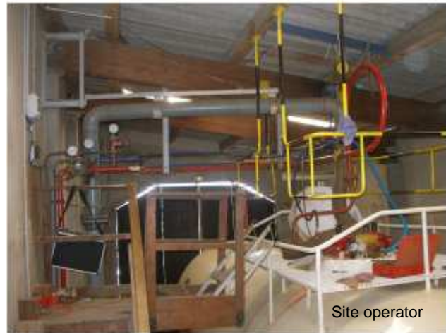
Chlorine tanker car transfer station (chamber no. 2)
