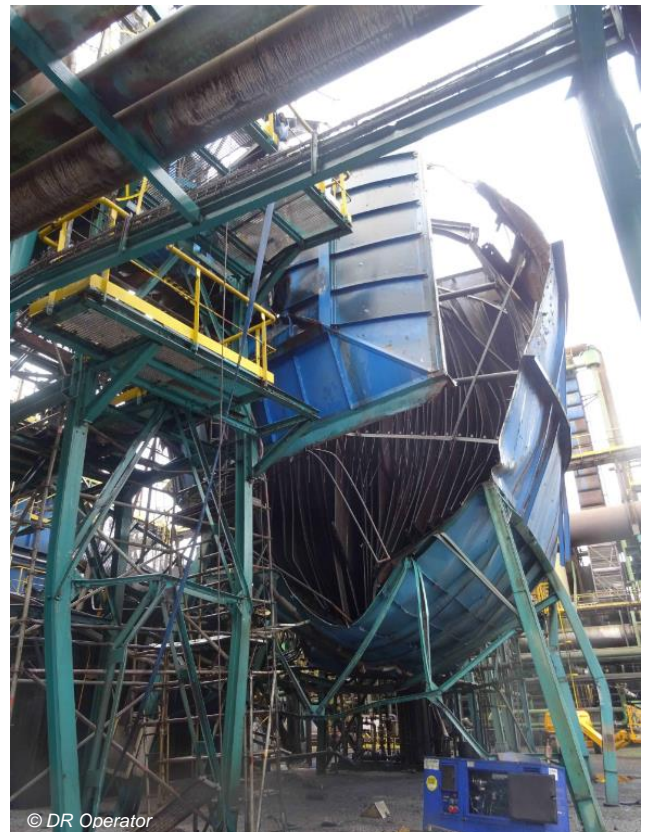
Figure 6: Condition of the tar extractor DE3 after the accident
