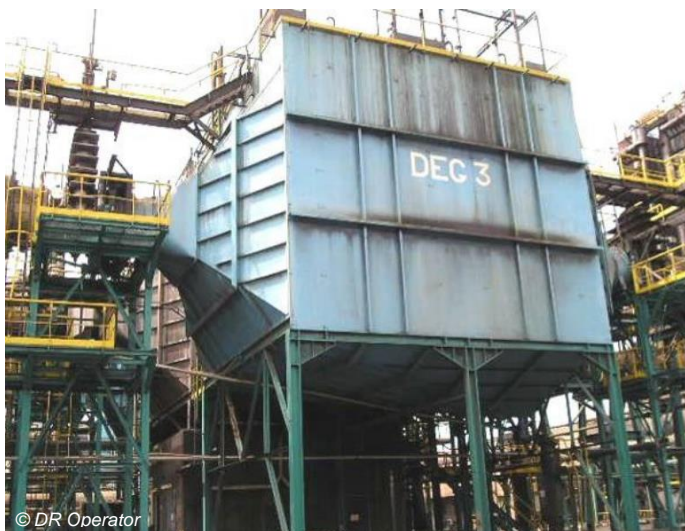
Figure 5: Initial state of tar extractor DE3 before the explosion
