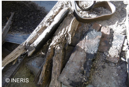
Pieces of wood trapped in the hopper
