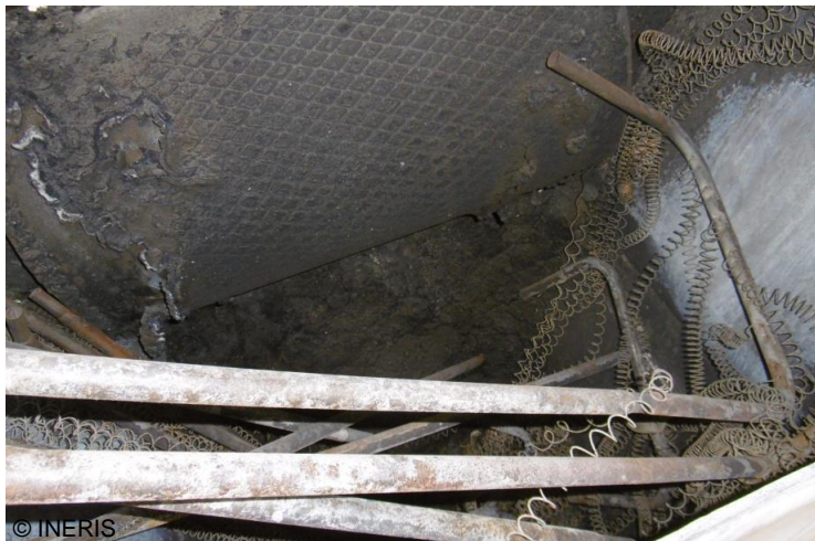
Upper part of the hopper
