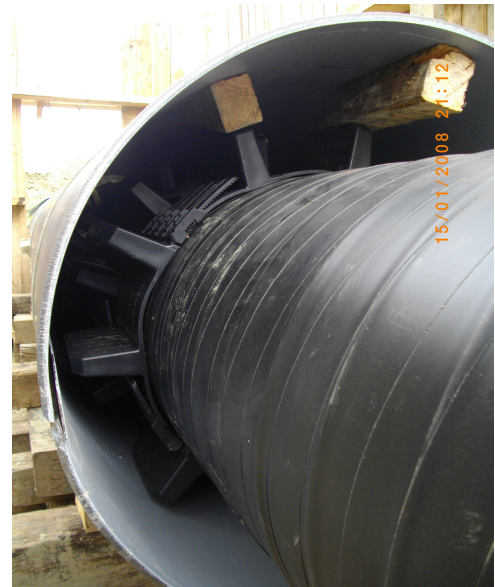
Copyright: Pipeline operator
