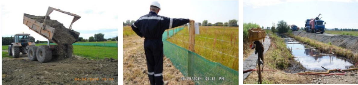
Copyright: Pipeline operator
