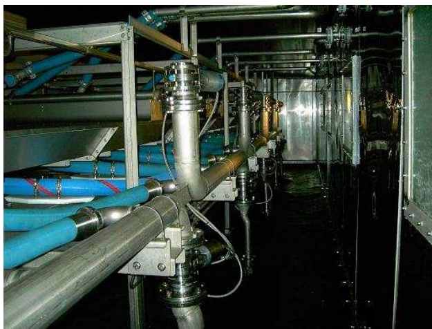
View of the filter inside the enclosure
