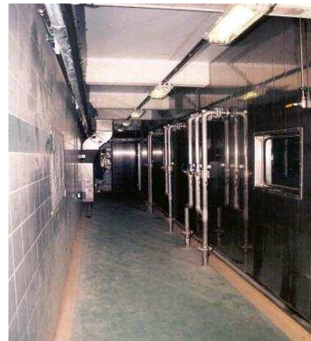
Outside view of the steel plated enclosure
