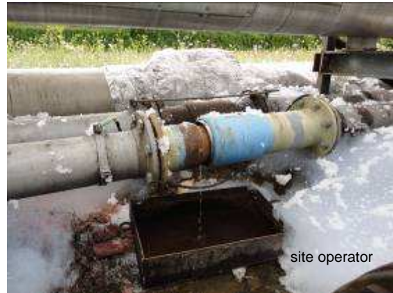
Damaged expansion compensator
