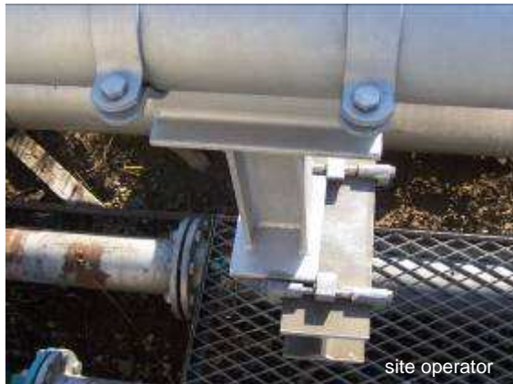
Dislodged pipe bracket
