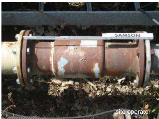
Expansion compensator before the accident
