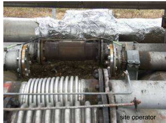
Expansion compensator taken apart after the accident
