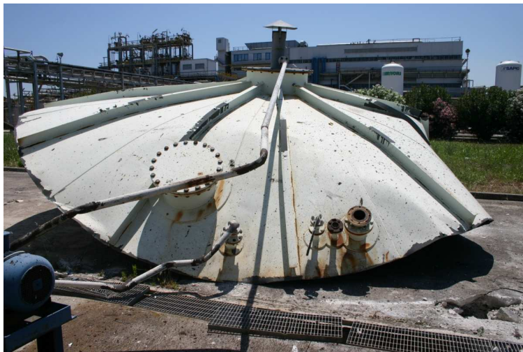
Fig. 9: Exploded roof, note the absence of plain flange on the air line (source: ARPA Puglia)
