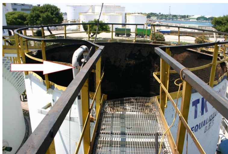
Fig. 5: Pulled-off sparger line on the TKX viewed from the walkway (source: ARPA Puglia)
