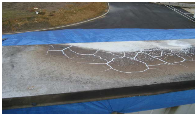
Close-up of property damage (source: DREAL)
