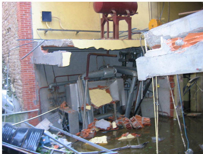
Press room damaged by the explosion (Source: site operator)
