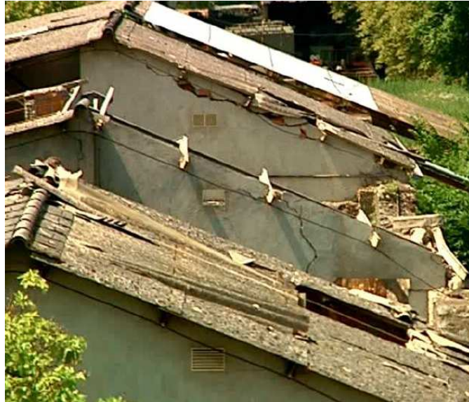
Destroyed roof on the premises (Source: site operator)
