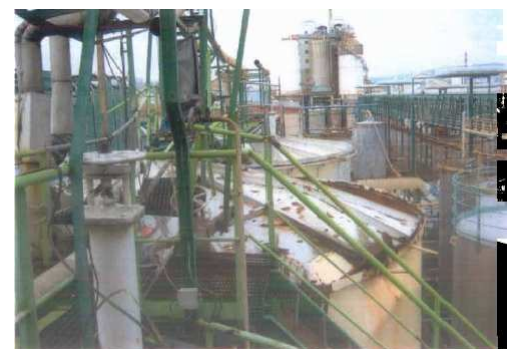
The dome of the storage tank is partly opened around the circumference.
