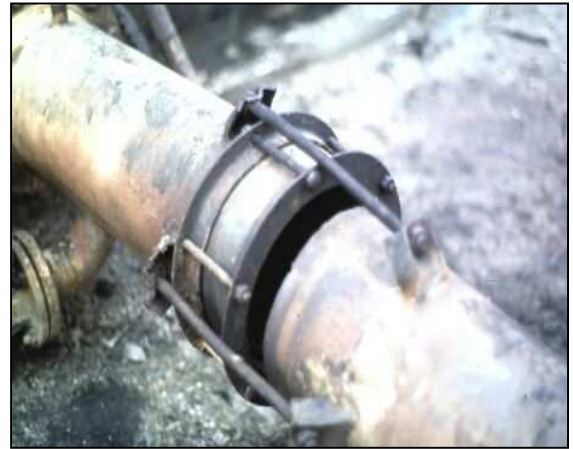
Union responsible for the leak
