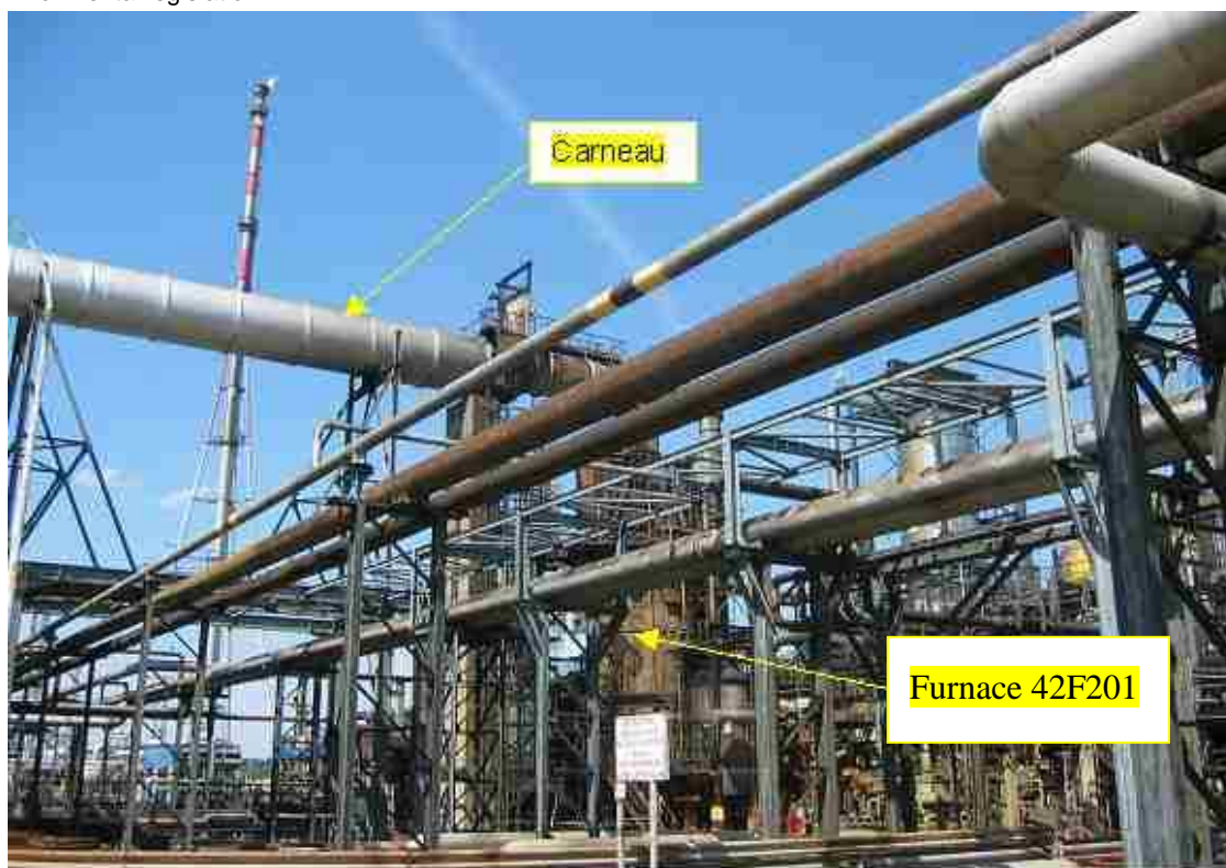
Overall view of the HDS unit (after the fire)
