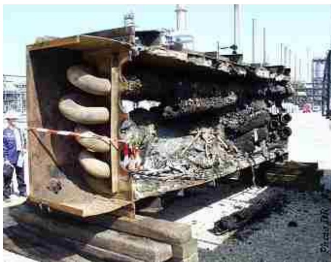
Partial view of furnace 42F201 after the fire and dismantling for inspection
