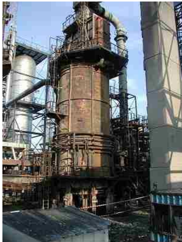
View of furnace 42F201 (after the fire)
