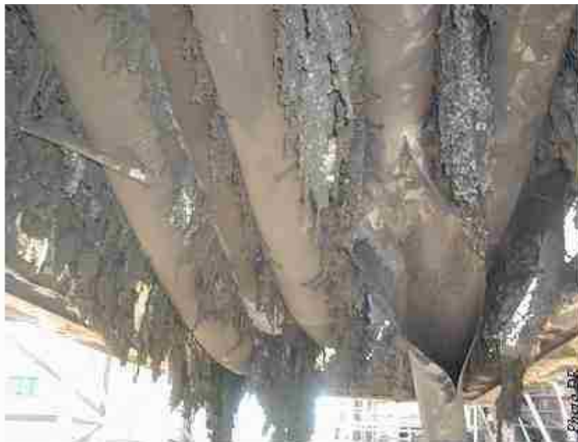
View of the lower convection layer (after the fire)
