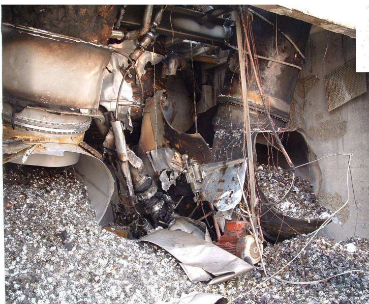
Damaged columns filled with catalyst
