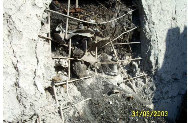
Machine impact in concrete wall
