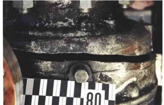
Photo: DRIRE Ile-de-France
