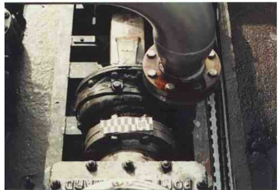
Photo: DRIRE Ile-de-France
