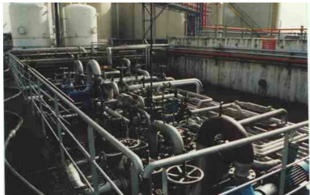
Photo: DRIRE Ile-de-France
