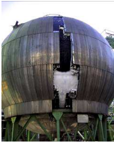
Superficial damages suffered by a NH 3
