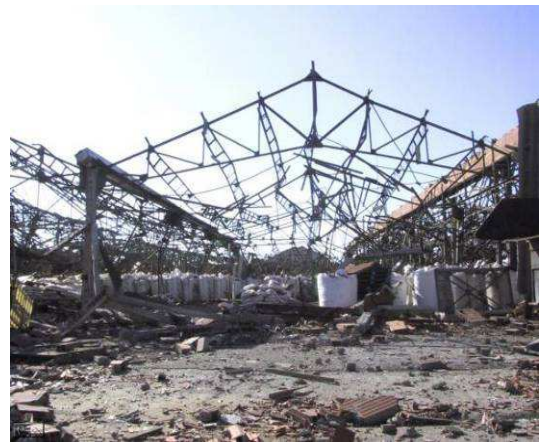
Warehouse destroyed by the blast
