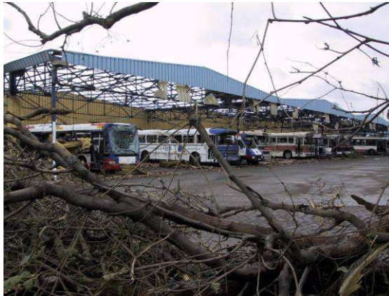
Bus depot destroyed
