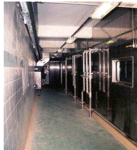
Outside view of the steel plated enclosure (RR)
